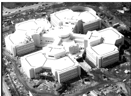
1995: Construction of Division XI Maximum Security wing of Cook County Jail - a $95 million, 1,600 prisoner facility.
